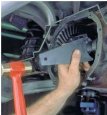
P35-7 Using the proper tool, drive the shims into position until they are fully seated.
