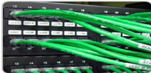
Front of Patch Panel
