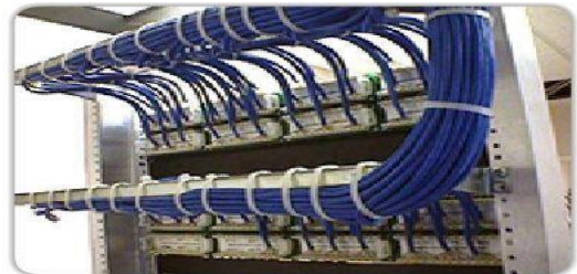
Rear of Patch Panel
