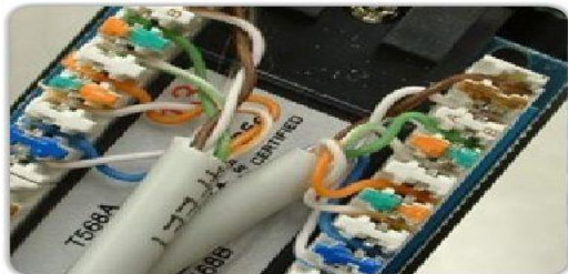
Close Up of Back of Patch Panel
