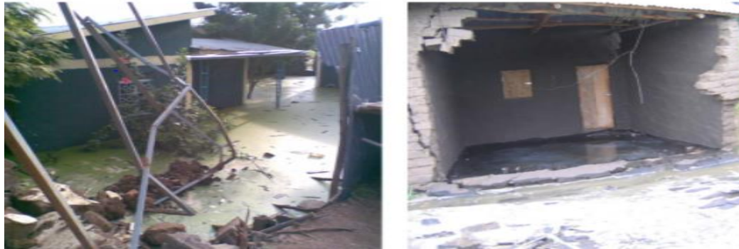
Figure 1.5 Homes damaged by the 2006 flood in Gambela town, Ethiopia.
